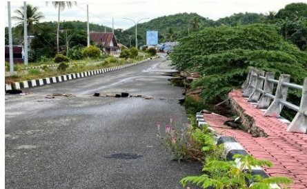
Figure 1. Damage Conditions at the Study Location
