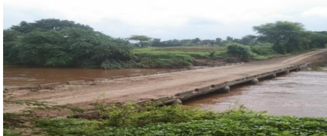
Figure 9: During flooding , the height of the bridge from the water level that caused danger to passers
