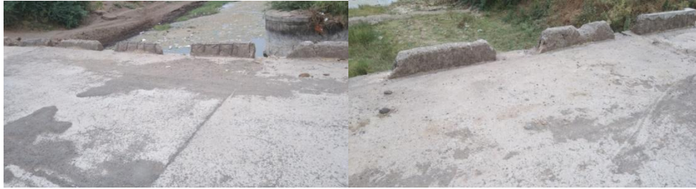
Figure 6: Damage Wheel Guard and Reflectors
