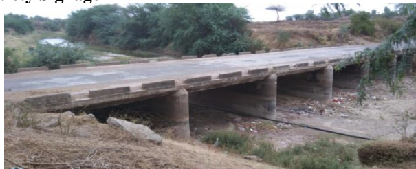
Figure 9: Lack of Lighting and Safety Signage
