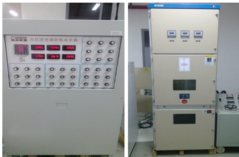
(a) Load cabinet
